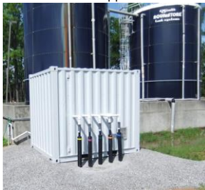
Above, a look at the leachate pumping system. Right, Brad Granley shows just how high the grass can grow.
